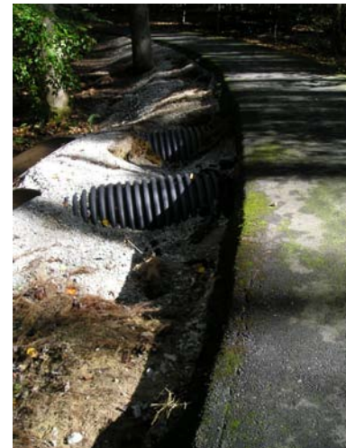
Tropical Storm Lee damage to Mason Neck Bike Trail near the Woodmarsh Trail Parking Lot.
