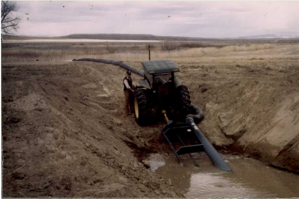
Tractor powered Gator pump, diverting water from the river (top), and the Leota drain (bottom) into the L-10 unit of the Leota Bottom.
