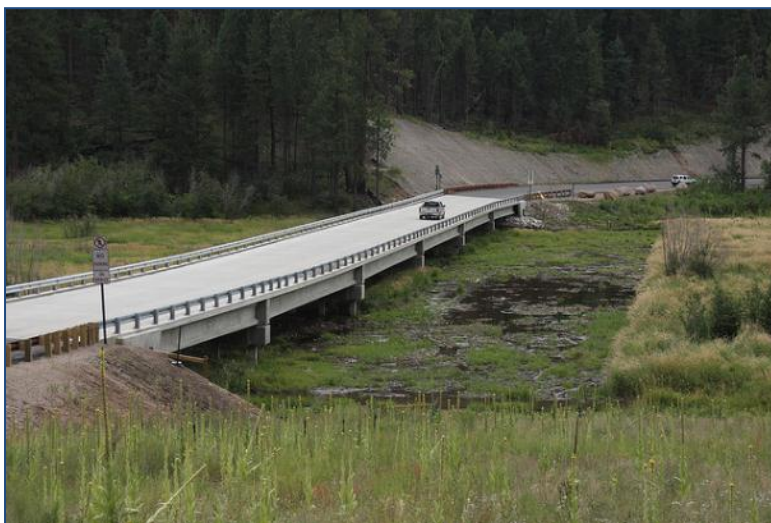
Figure 28. Newly constructed bridge on Highway 126, Jemez Mountains, New Mexico (photo courtesy of J.N. Stuart).
